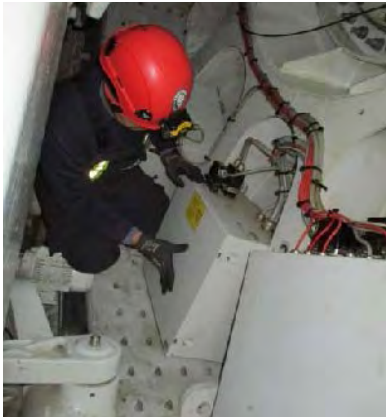
Working on Rotor Control Box
