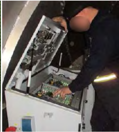
Nacelle Control Panel
