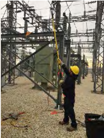
Grounding using a hot stick
