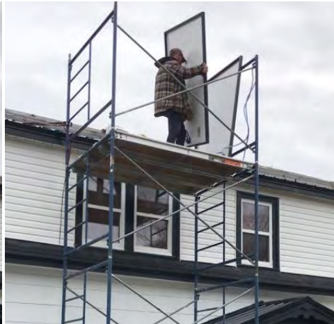
Stacking groups of solar panels and securing to scaffolding for eventual placement
