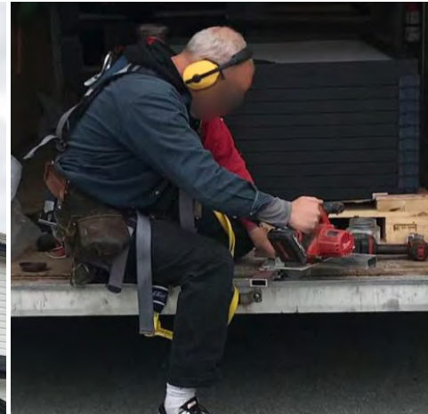
Using circular saw to cut a length of rail in the fabrication of a rail extension
