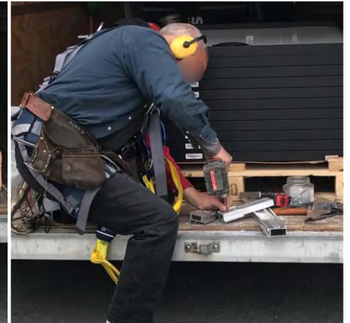
Using driver to a self-tapping screw into a splice block that attaches to the pre-cut rail section in the fabrication of a rail extension
