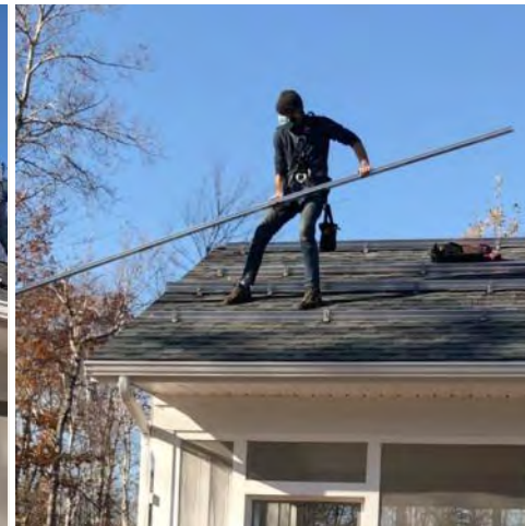
Lifting a rail that will be attached to a series of L-brackets protruding from roof
